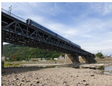
Fig. 1: Railway bridge crossing the Elbe in the city of Ústí nad Labem
