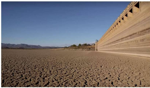
Fig. 1: Empty Nqweba Reservoir due to reservoir sedimentation (2019)
