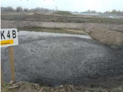
Fig. 1: One of the dewatering ponds after having been filled with dredged sediment.
